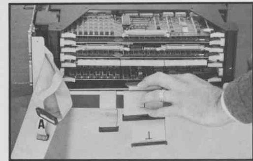
Figure 55 Short Tape Control Cable [A] 10 mbit Ethernet cable
